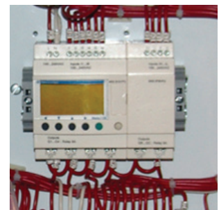
Programmable "smart" relay adds diagnostic and troubleshooting capabilities
