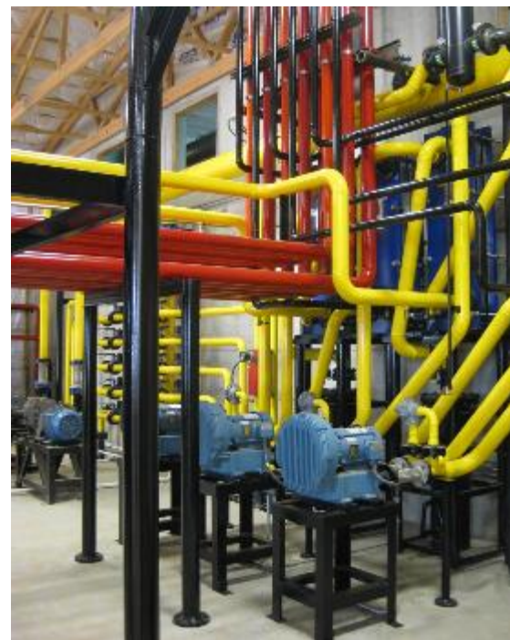
DVO Mixed Use Digester
